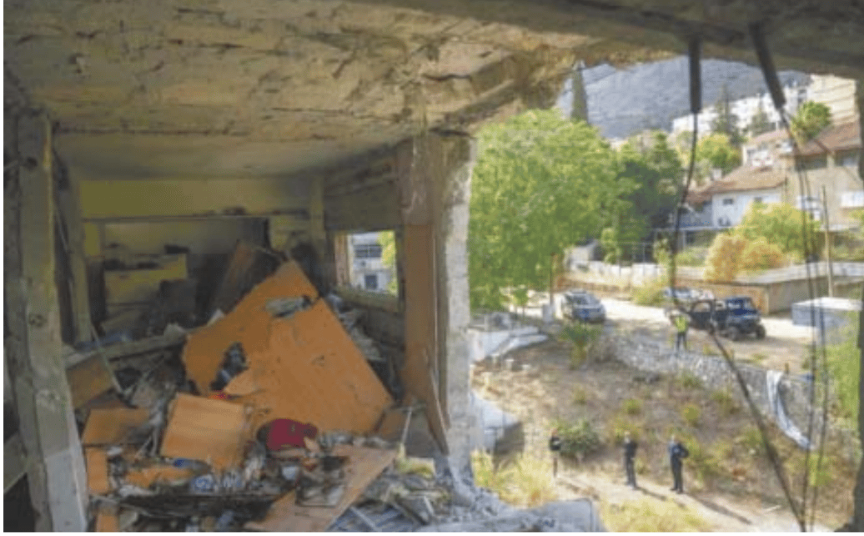
The site where a Hezbollah rocket hit a residential building in Kiryat Shmona, last year.
